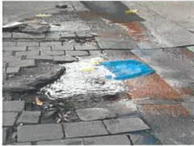
Before: leaking water meter
