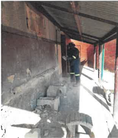
Before: peeling cement
