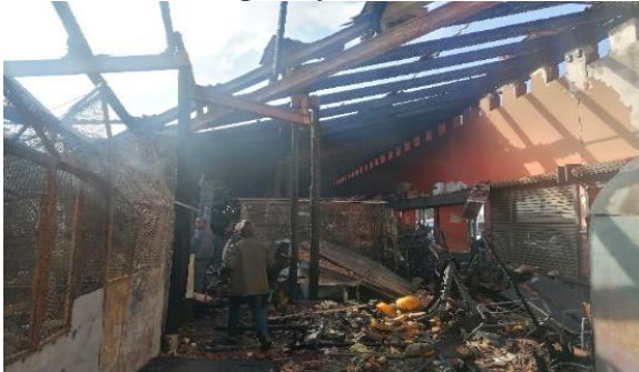
Picture 1 - Damaged by inferno
