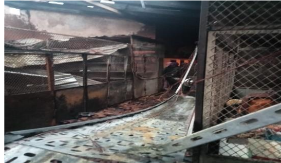
Picture 2 - Damaged stall
